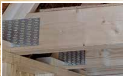
Plated Loft Joists
